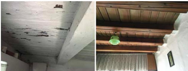
Figure 12: Left: ground floor-first floor structure (in the kitchen of the ground floor unit); Right: first floor-garret (divanhana ceiling)
